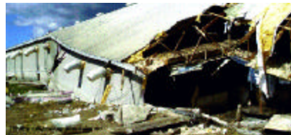
Innerkip - Summer 2001 - 12-year old deep-pit barn Severe corrosion of cement pillars above liquid
