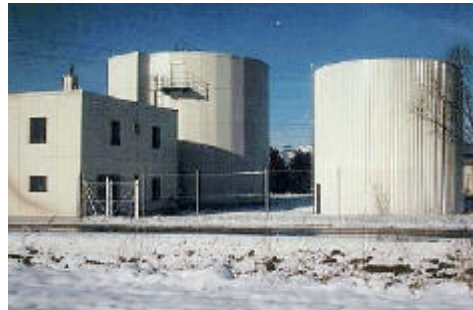
German GBU mixed manure-waste digester 3,000 cu.m./yr - hydraulically operated, continuous flow (Canada - Rentec Renewable Energy)
