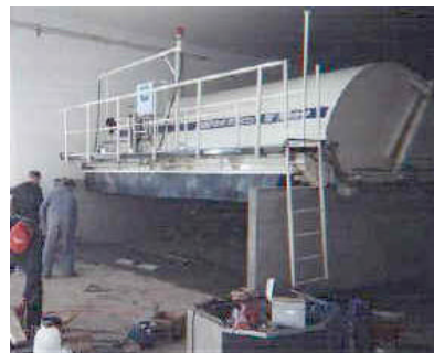
Transform Composting – Abbotsford, BC Covered building - controlled
